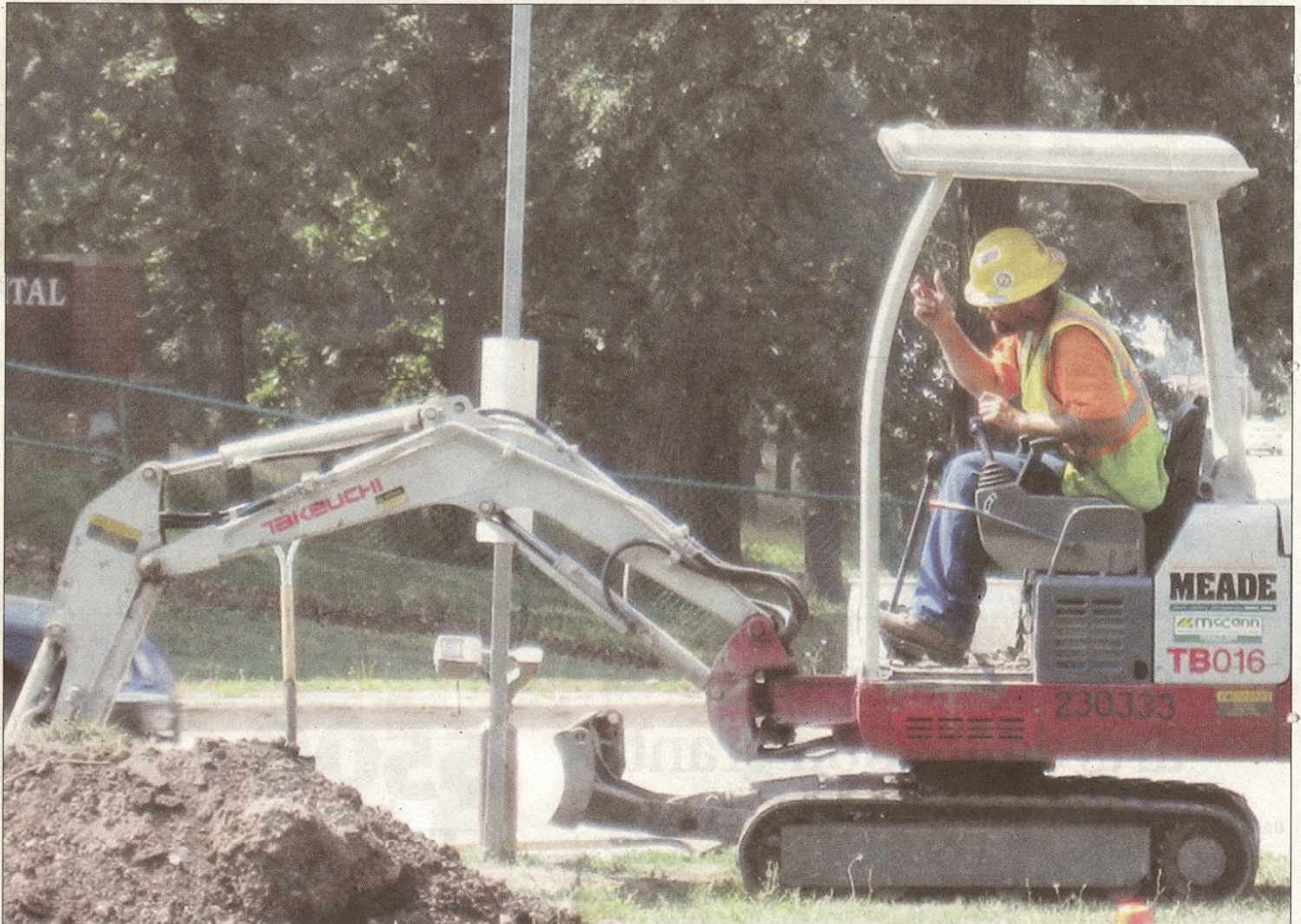
Construction crews install red light cameras at 159th Street and Cicero Avenue in Oak Forest. MICHAEL DRAKULICH — SOUTHTOWNSTAR
